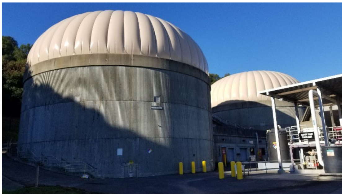
New covers for Digester No. 1 and 2
