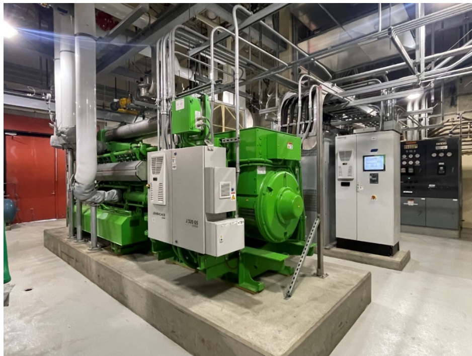
New cogeneration engine
