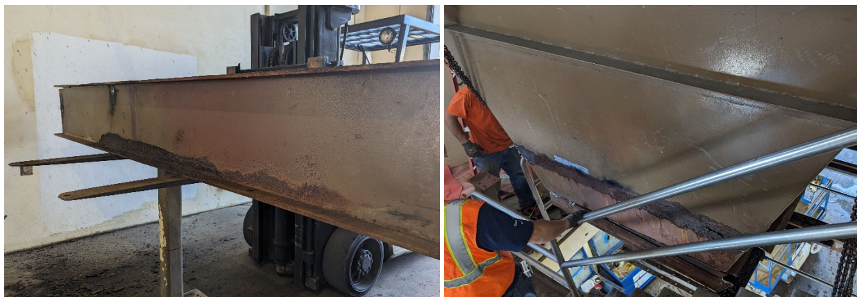
Corroded beam and side of biosolids hopper
