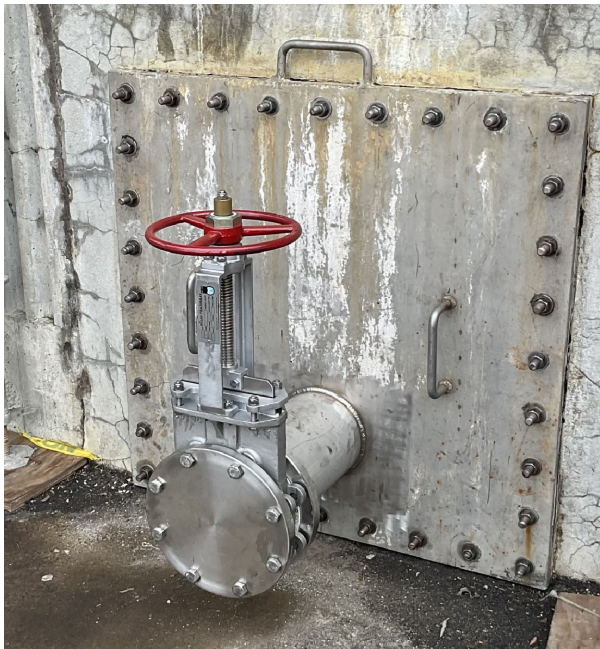
Emergency Drain Valve on Digester No. 2
